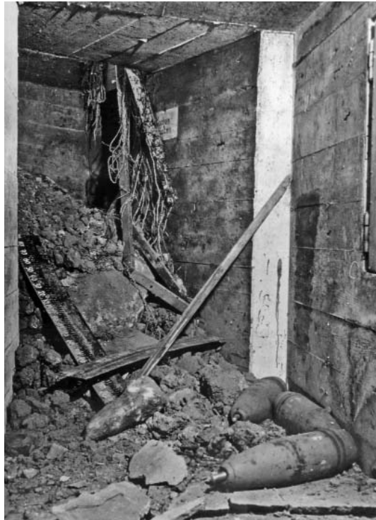
The reinforced bunkers could withstand hits by 500lb bombs, but special armor-piercing bombs could cause penetrations. This is the interior of one of the ammunition bunkers after a partial penetration and wall collapse. (NARA)
